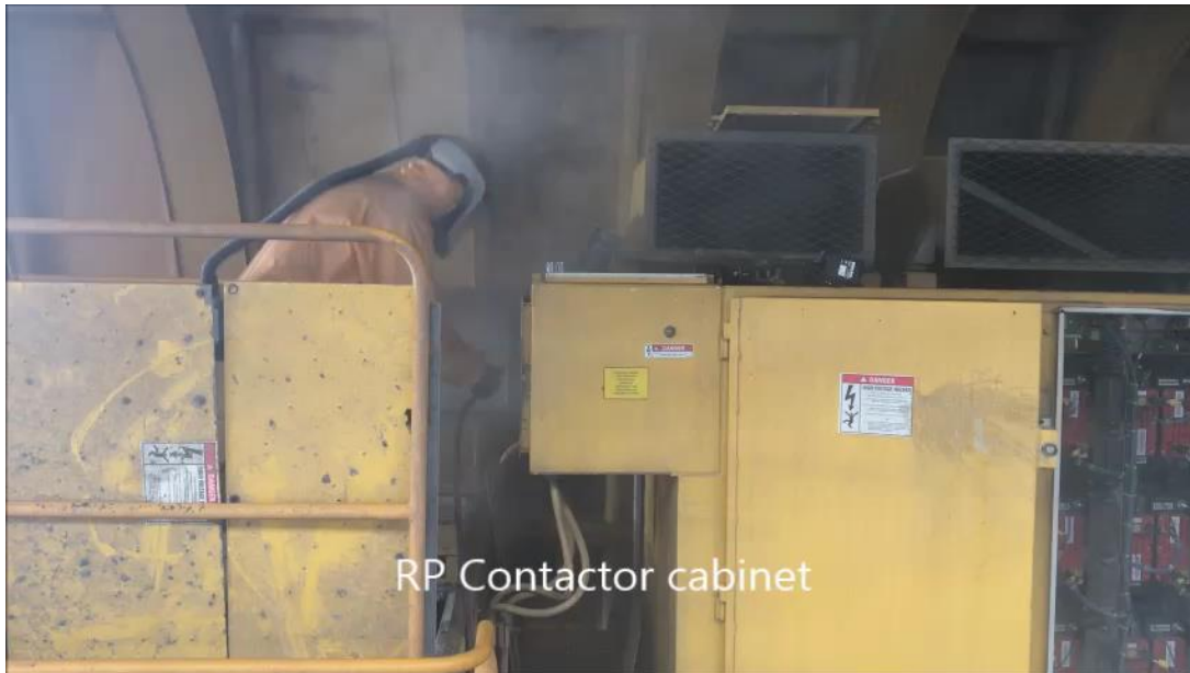
Figure 6 - Example of traditional compressed air cleaning of Komatsu 960E truck electrical cabinets
